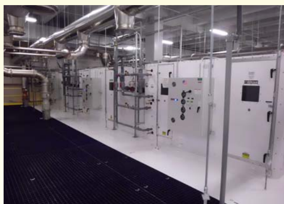
The air handlers and walkable surface above the clean room. The clean room is hanging from the second floor ceiling on threaded rods.
