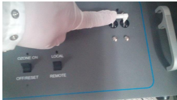
Main power switch turned ON for ozone generator
