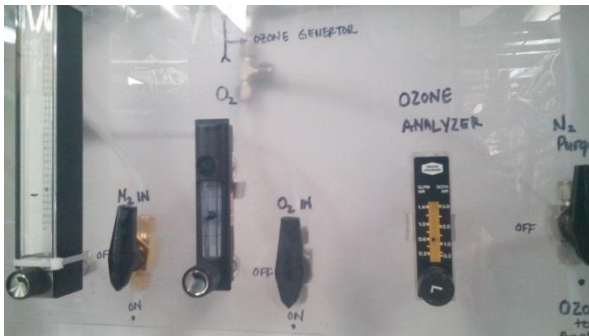
Gas valves are on – all pointing downward
