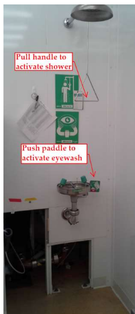
Keller Hall emergency shower-eyewash station
