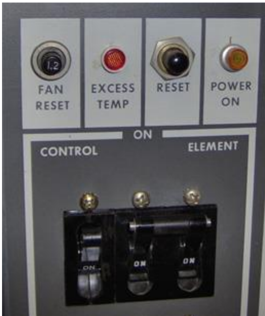
Fig. 4 Main power Control & Element switches.
